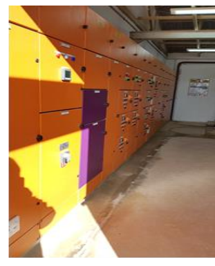
MCC Control Panel
