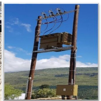
Bulk Electrical Supply
