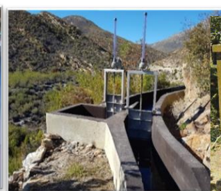
Barrydale bulk water infrastructure
