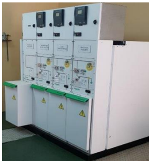
Swellendam Water treatment works- High Pressure Filter
