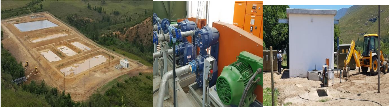
Suurbraak WWTW and Bulk Water Scheme Phase 1 upgrade (first portion); Water System upgrade
