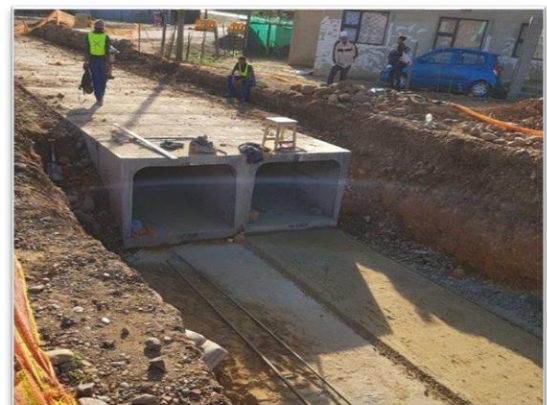
Railton upgrade gravel roads and stormwater phase 2: Gazania Street, Vygie Street, Kossmos Street, Tulp Street
