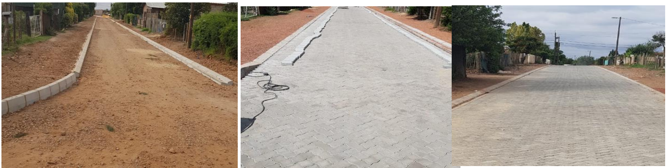
Phase 2 of the Railton gravel roads and stormwater channels upgrade, as well as the upgrade of
