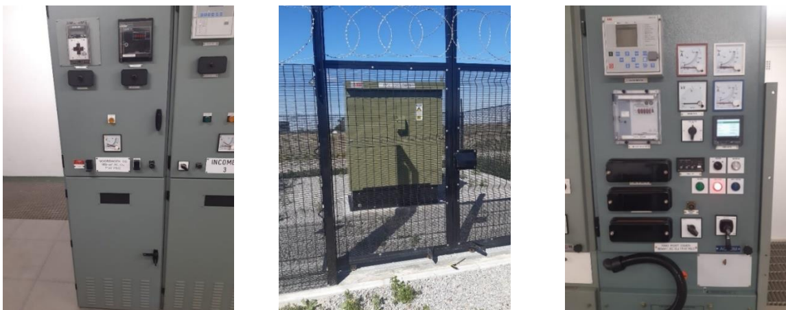
Images above (from left to right): Noordhoek Substation, New Port Owen Ring Main Unit (RMU), Port Owen integrated into main feeder.
