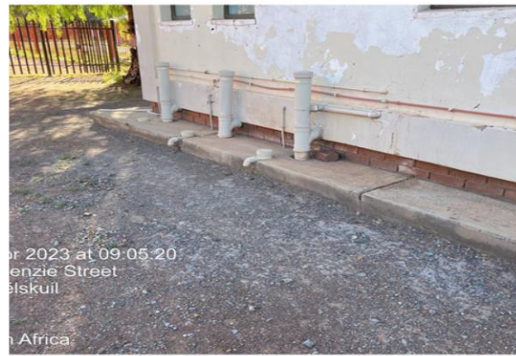
Photo 9 Worn-out paint at Municipal Library
