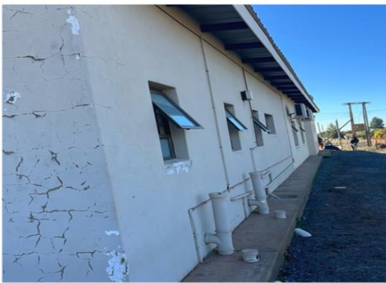
Photo 7. Worn-out paint at Municipal Library
