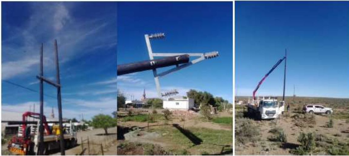
MV transformer platform and intermediate pole with A-Frame
