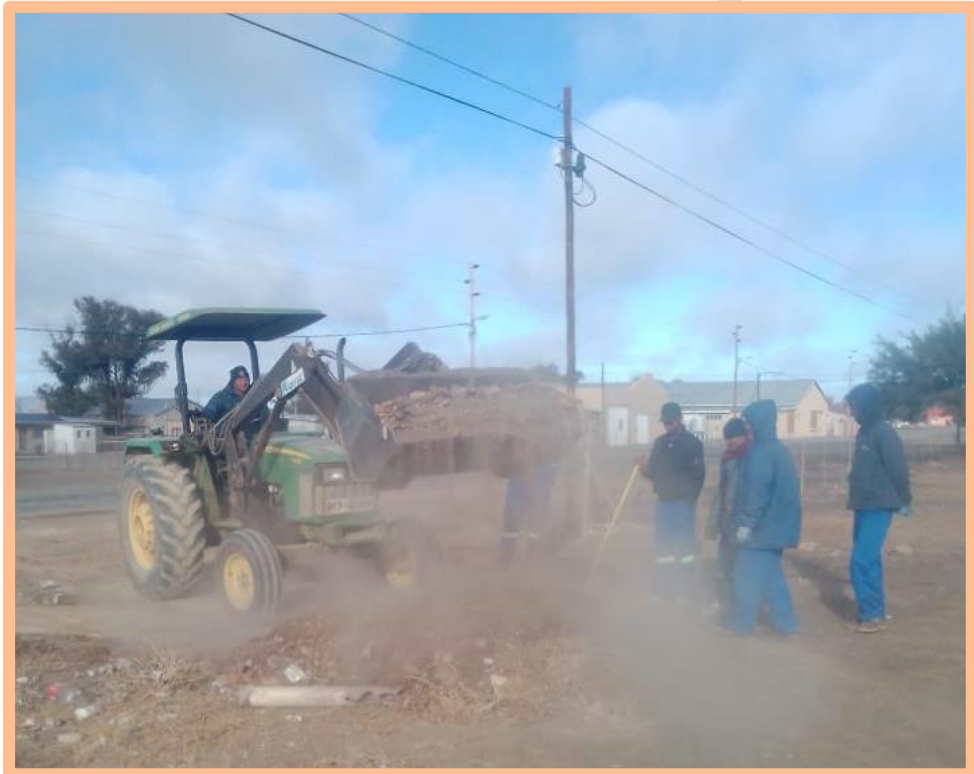
Pictures 8: Removal of illegal dumping
