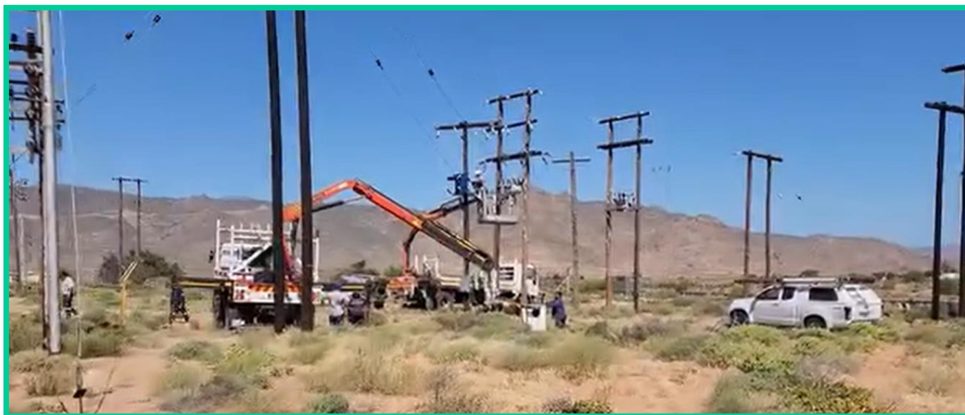
Picture 17: Electricity transformer installation
