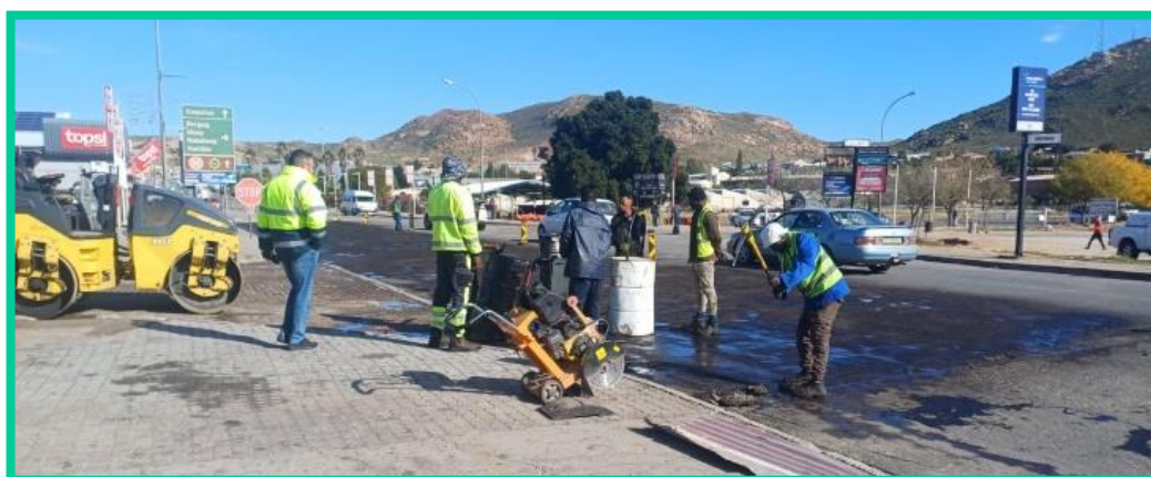
Picture 26: Slurry and tar Voortrekker Street, Springbok CBD
