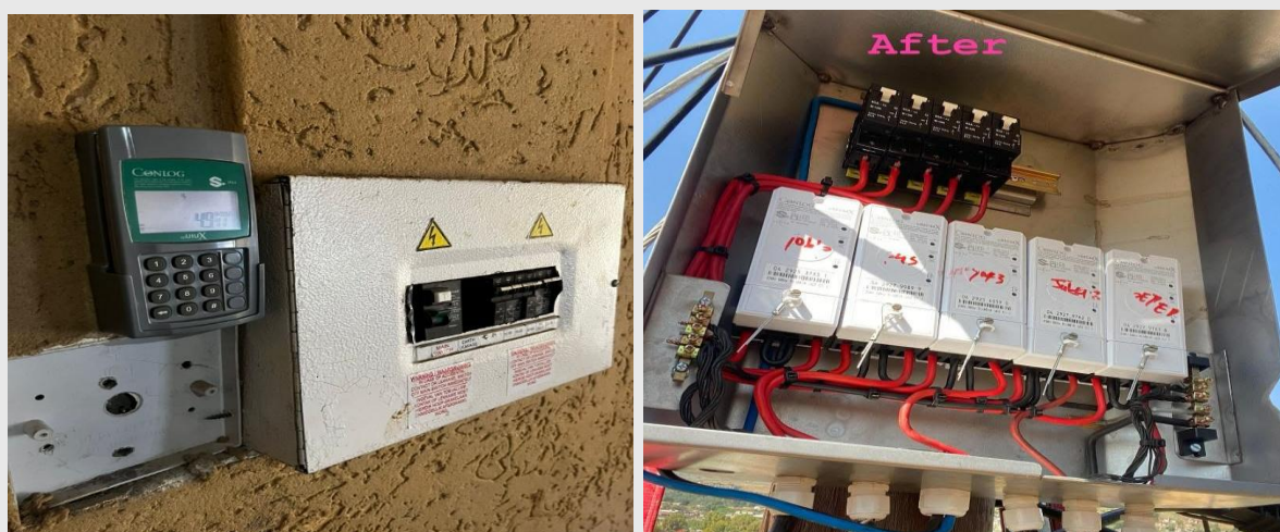
Figure 17&18: Installed Smart meters and keypad
