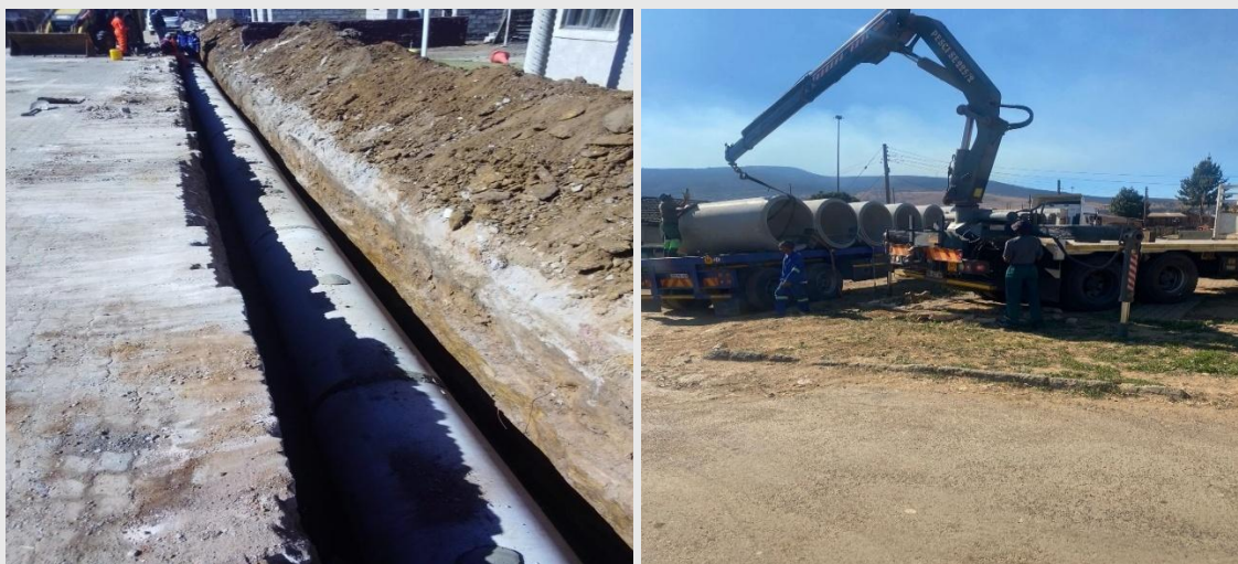
Figure 24&25: Mongwe stormwater and Slahle Stormwater pipes
