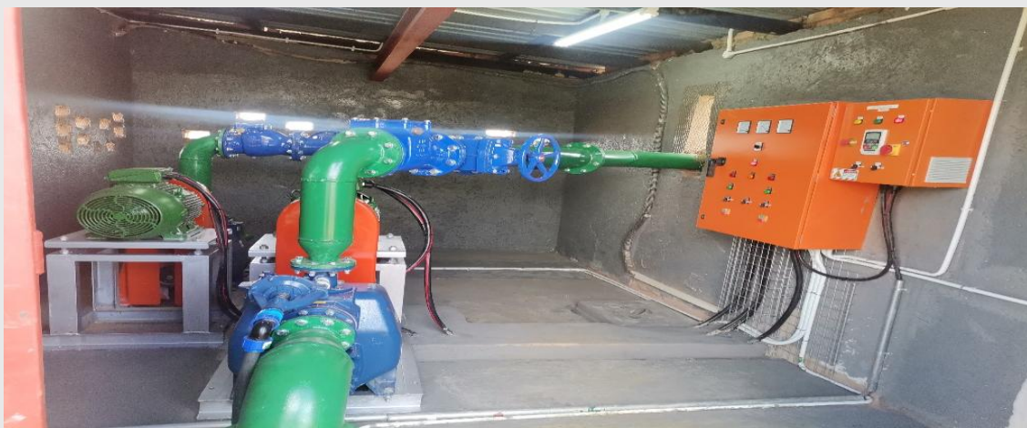
Figure 10: Mechanical and Electrical Components
