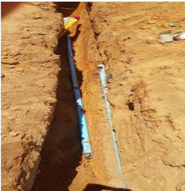
Fig 1: Damaged 75mm existing water line
