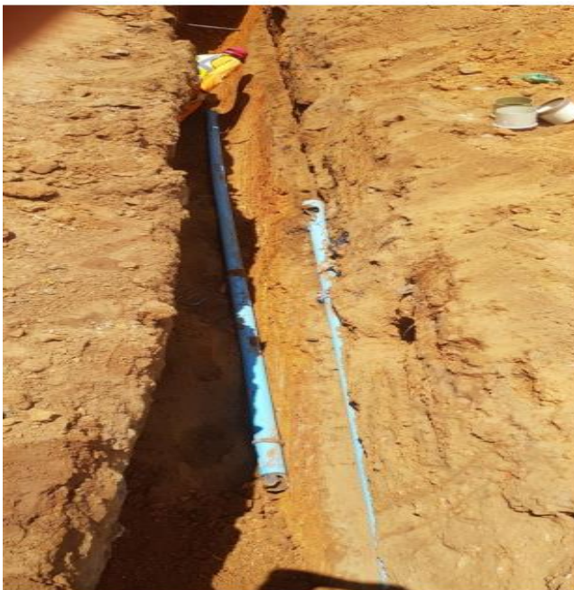
Fig 1: Damaged 75mm existing water line
