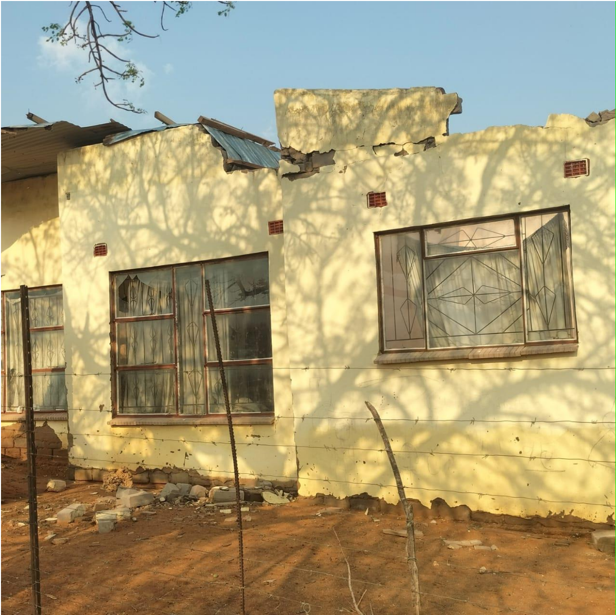
Roofing uprooted and family left stranded at Masea village in ward 08
