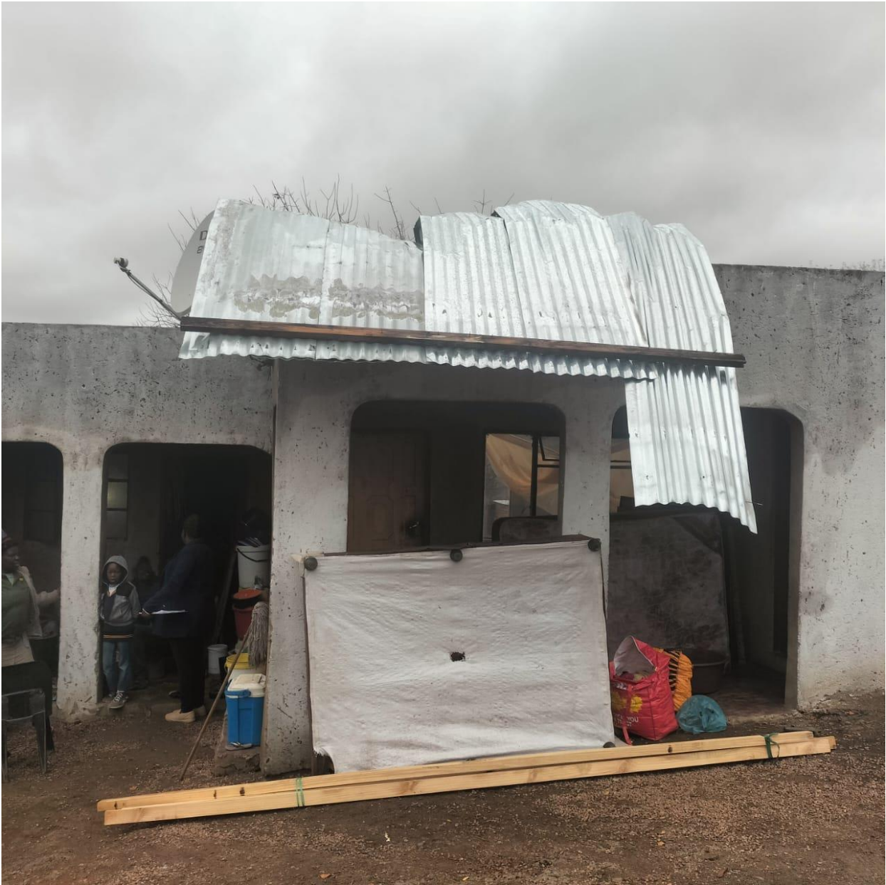
Roofing uprooted and family left stranded at village in ward 12
