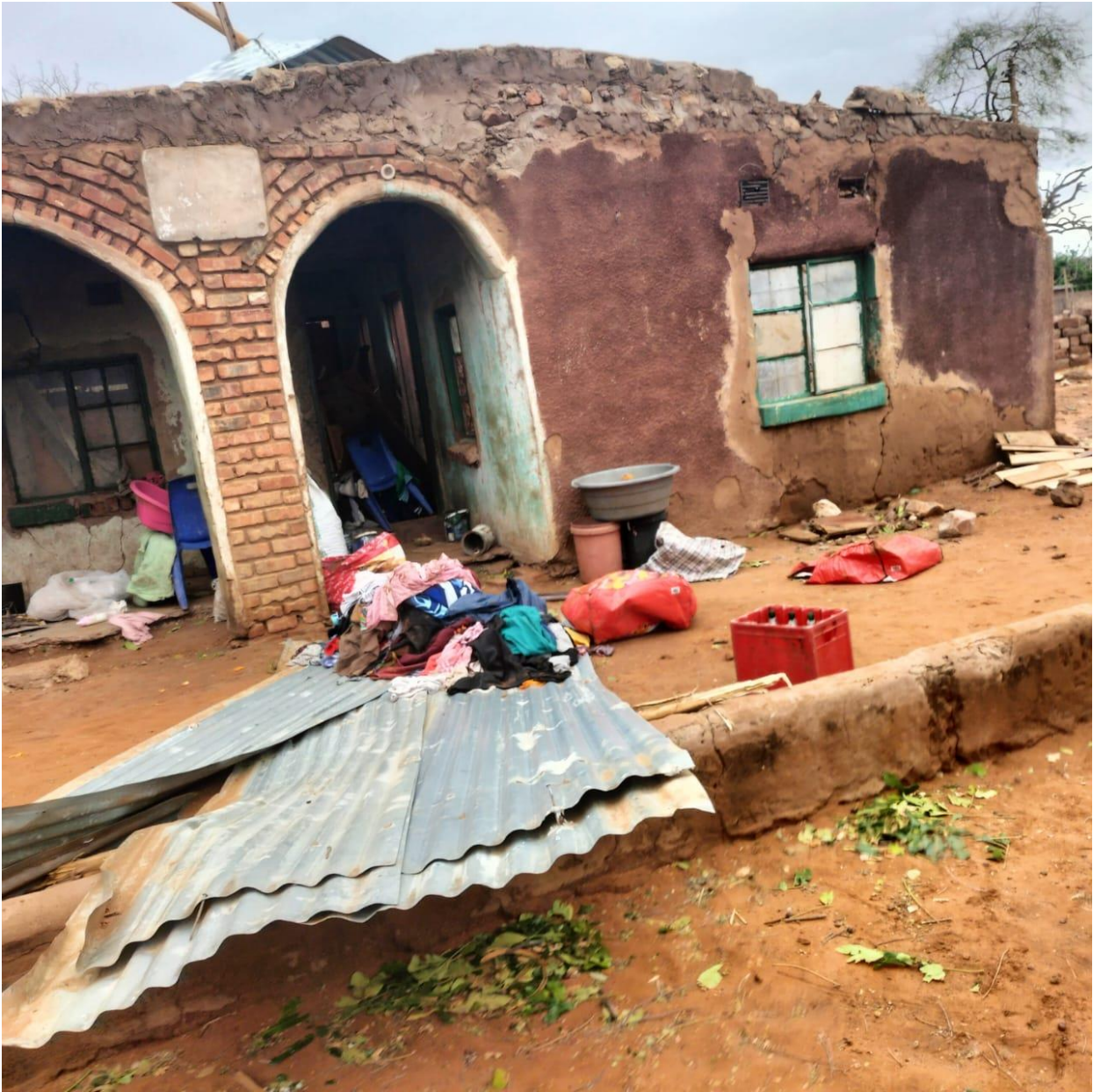
A roof was uprooted by heavy storm at Mabvete village in ward 08
