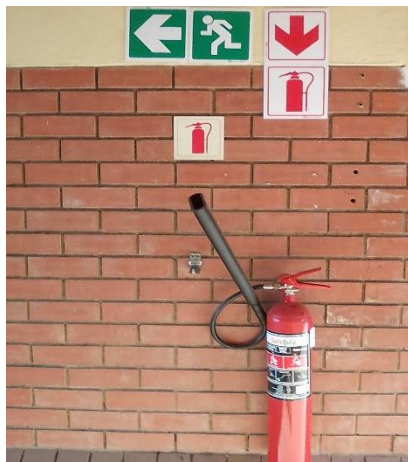
Valid fire extinguisher & SABS approved signage
