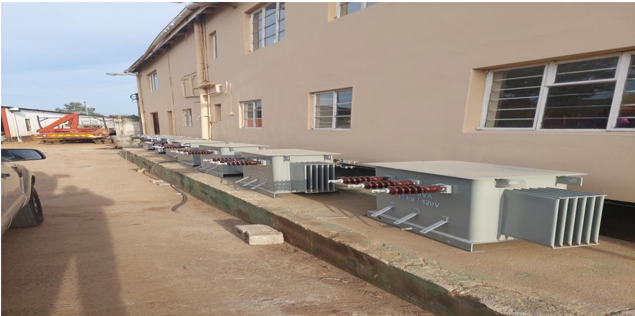
SUPPLY AND DELIVERY OF 1X500KVA (KOKSTAD CRU) MINI SUBSTATION
