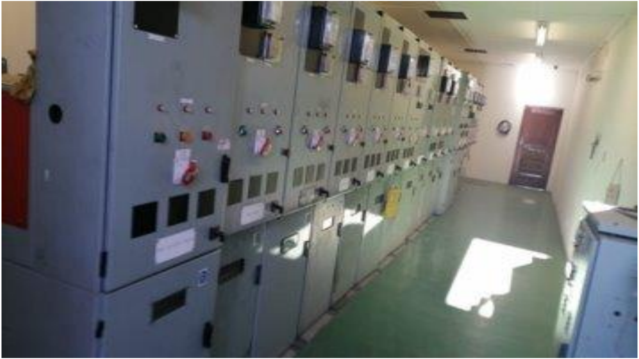
OLD JIMPAYNE SUBSTATION SWITCHGEAR
