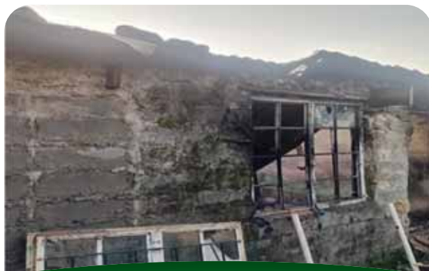
Conveys the aftermath following a structural fire incident in Ward 26 (eZihlabathini)
