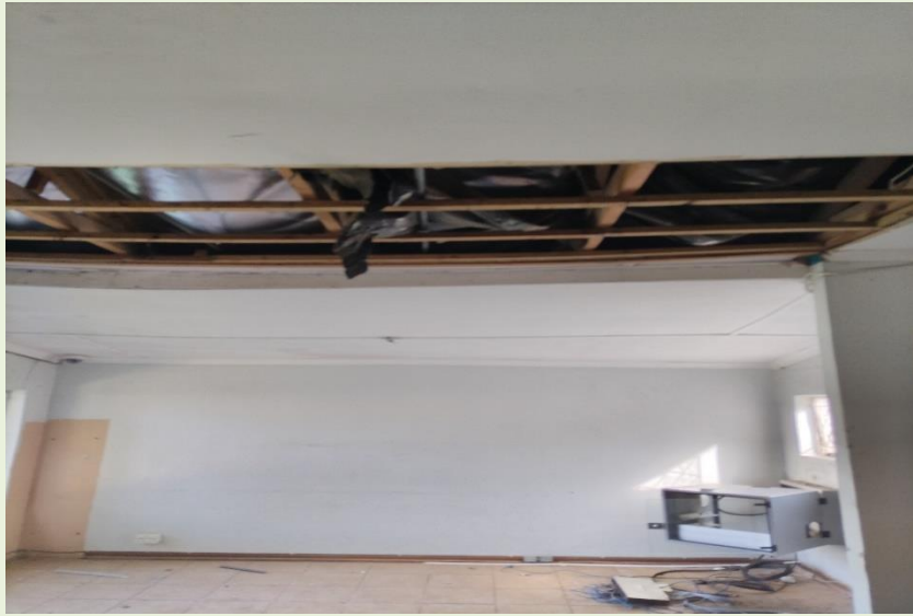
-Disaster Station before repairs and painting of the building.
