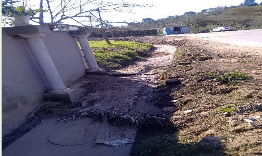
Unblocking of open drain in Thubalethu Township in Melmoth Town .
