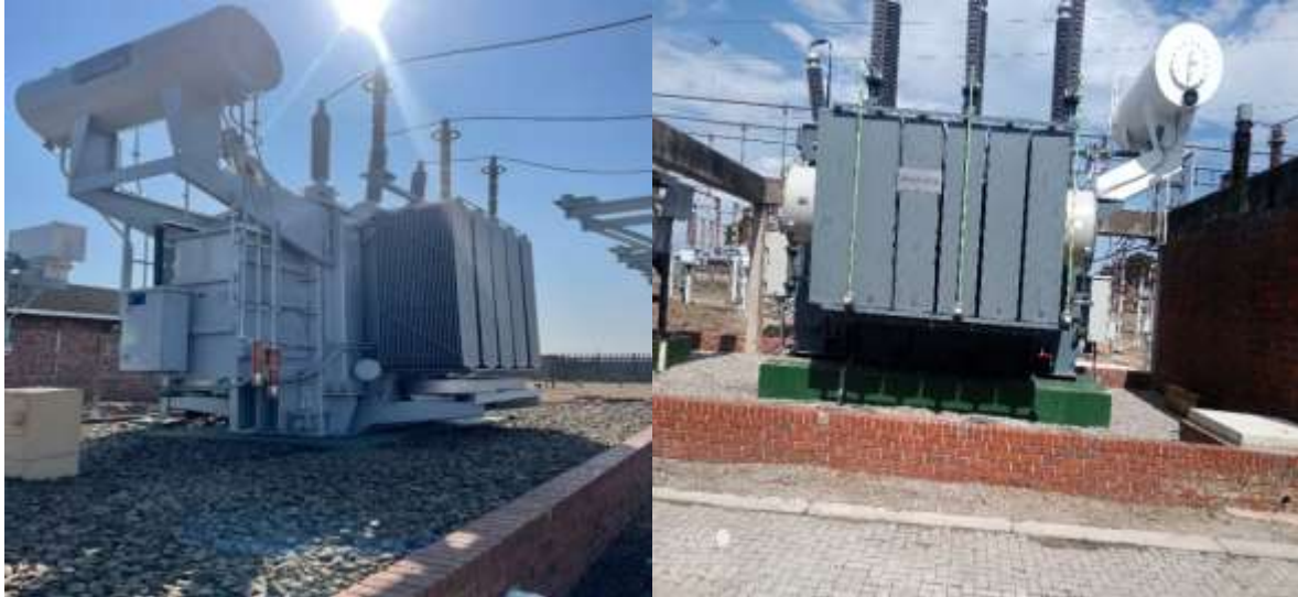
Picture **: Hercules Substation 2x 132/11kV 40MVA transformers installation: Ward 2; Co-ordinates: 28°44'58.4"S 32°02'40.6"E
