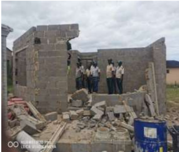
Inspection of unoccupied buildings / construction sites and removal of squatters is attended to by Vagrant and Squatting control team
