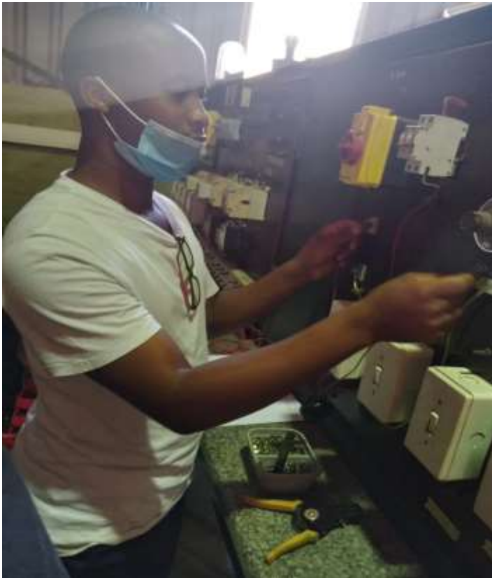
Figure 4 of 4: Basic electrical skills
