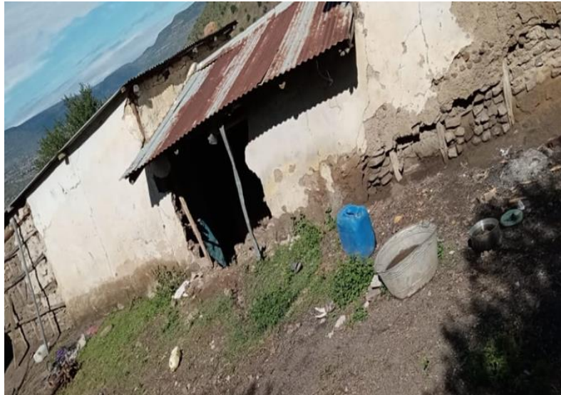
FIGURE 30: HOUSES DAMAGED AT WARD 16 KWA-GXOBANYAWO AREA
