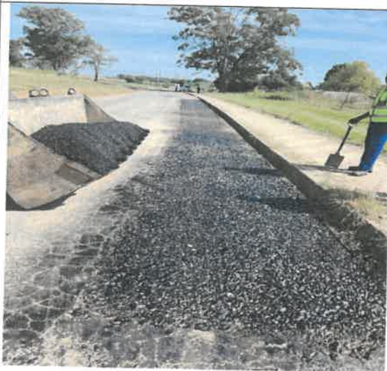
Figure 2 paving potholes in Bergville Tatham road.
