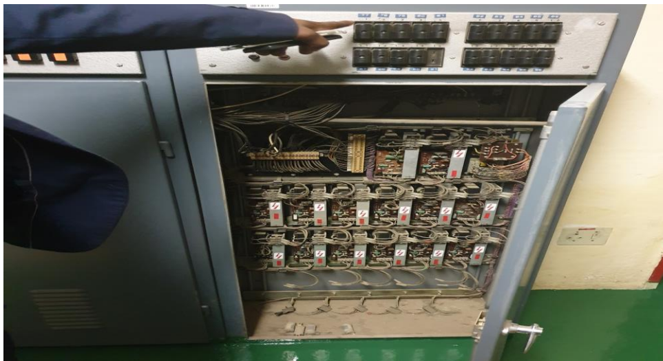
Figure 1: Old Power control rack
