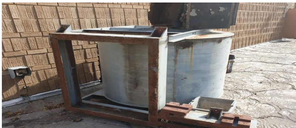
Figure 2: Old Air Condition system that need to be fixed
