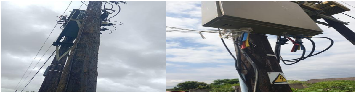
Picture 1: Cables cut from the transformer leaving customers in the dark
