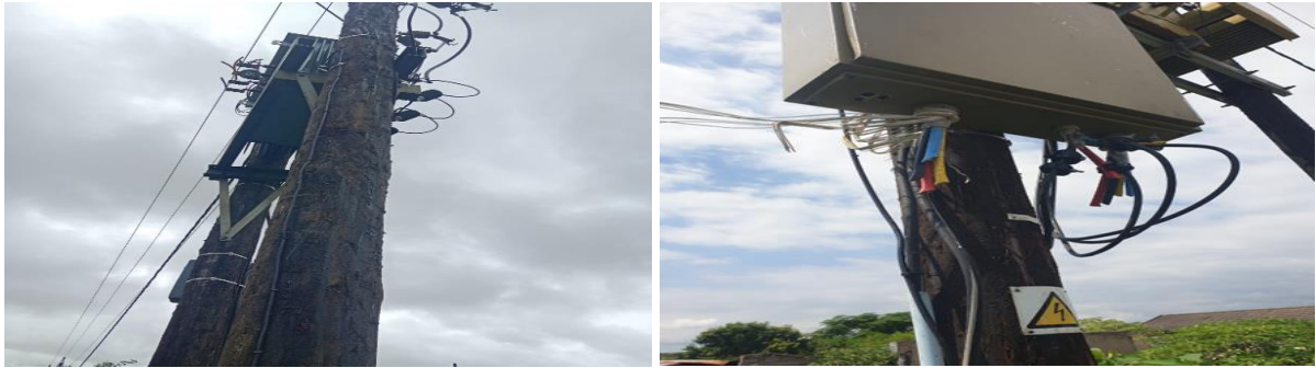
Picture 13: Cables cut from the transformer leaving customers in the dark
