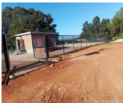
New sewer pump station Hankey
