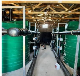
St Francis Bay new filtration plant.
