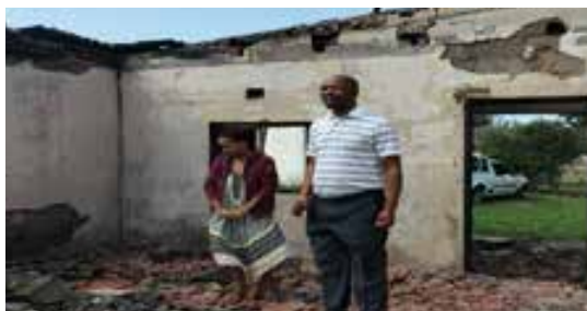
Photo 7: Denge family Roof blown off at ward 14 Khondweni area.
