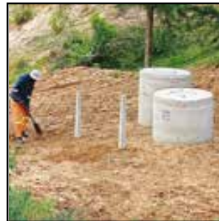
Photo 4: Pipe markers and Chambers
