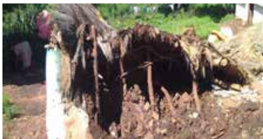
Photo 5: House damaged by heavy rainfall in ward 06 Mpendle area.
