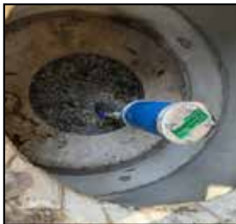
Photo 2: Air valve ring manhole
