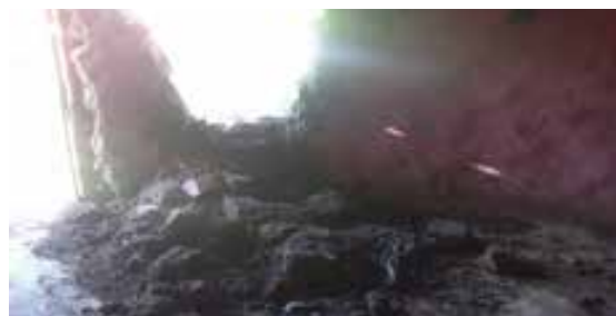
Photo 6: The house was damaged by heavy rain in ward 27 Mandawe area.
