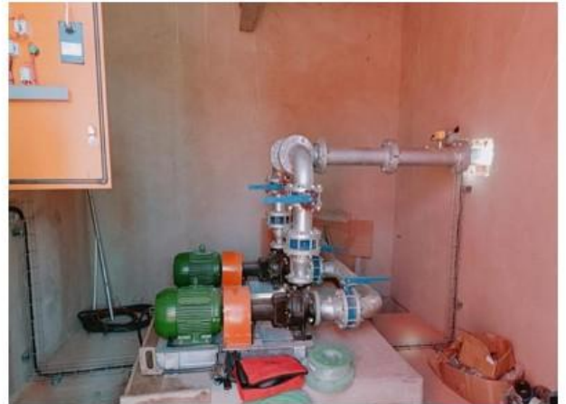
Pumps and Electrical panel
