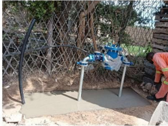
Commercial Meter installation
