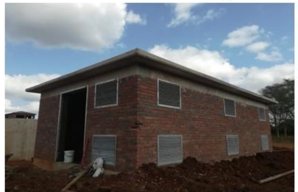
Clarifier – Pump Station
