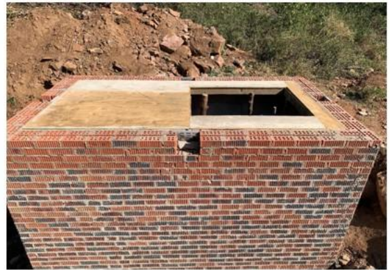
Inlet Meter Chamber
