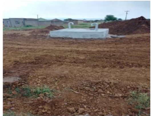
Air Valve Chamber
