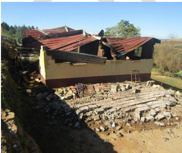
Structural fire at Mizpah in ward 10 at uMvoti
