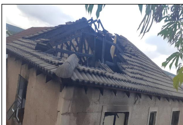
Structural fire on 17 th May 2021 at Greytown in ward 9 at uMvoti
