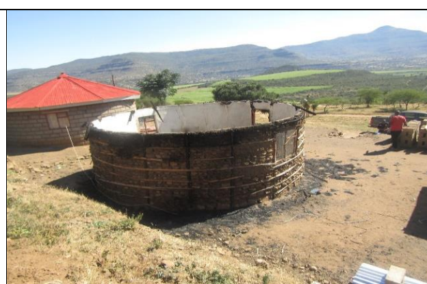
Structural fire on the 5 th May 2021 at Muden in ward 8 at uMvoti
