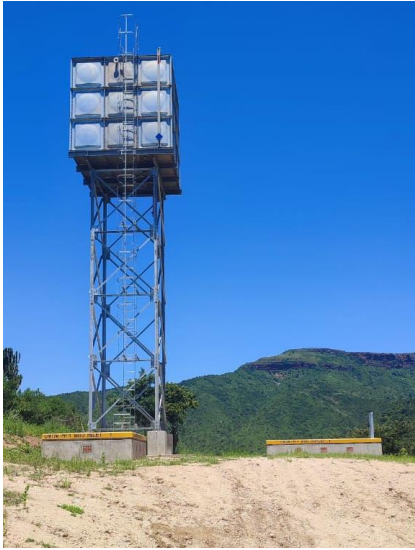
22KL Elevated Tank at Njengabantu
