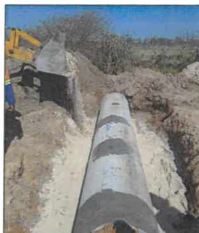
DR01129 (Protea Road flood damage repairs)
