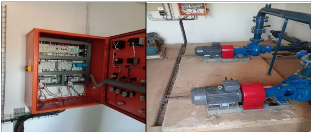
Nkwenkwezi Water Pump Station
