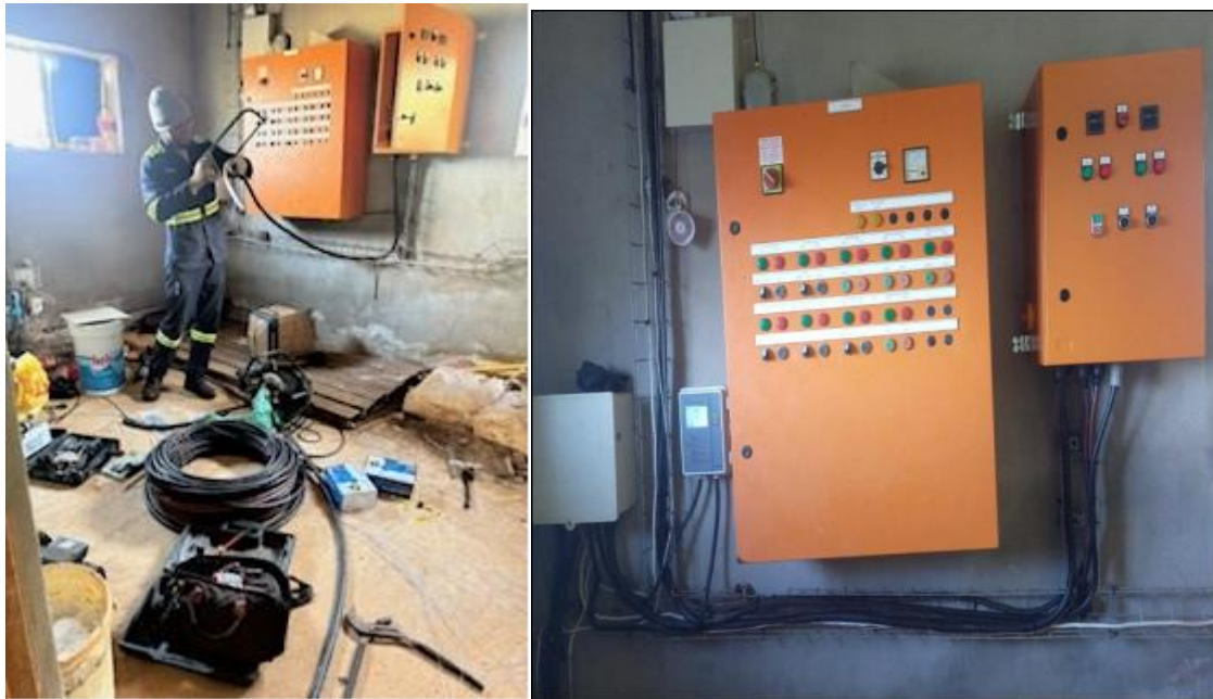
Clarkson Water Treatment Works
