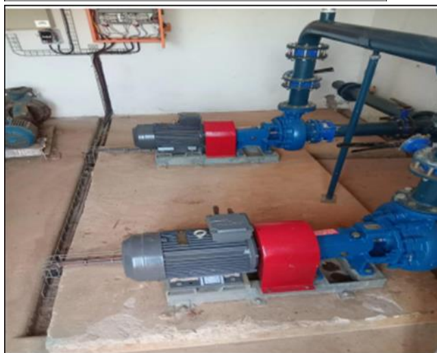
Nkwenkwezi Water Pump Station
