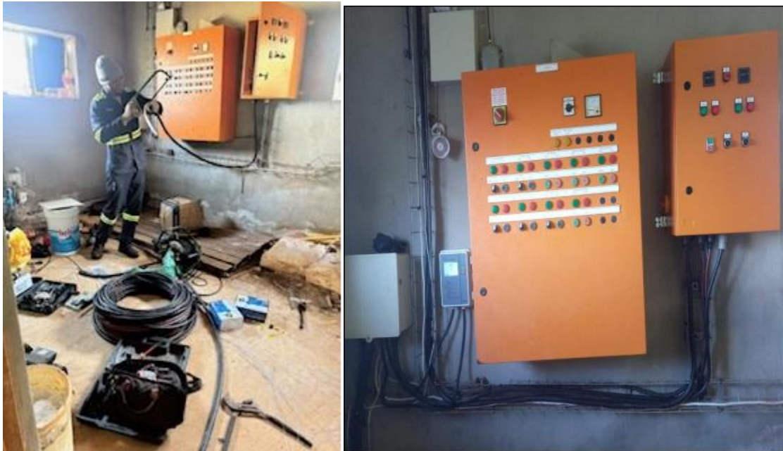
Clarkson Water Treatment Works
